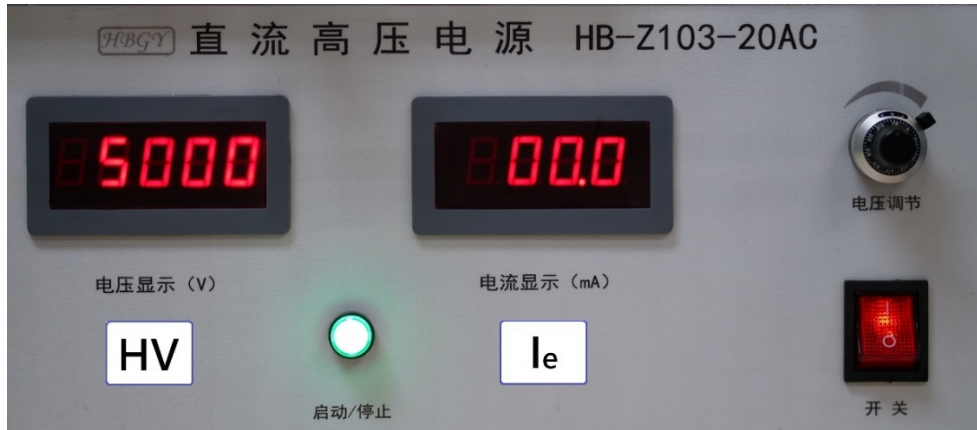
Figure 5.5: Measurement of HV and I_e on high voltage power supply.
